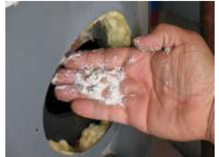
Installed 2/21/07 – room #27 still in service
