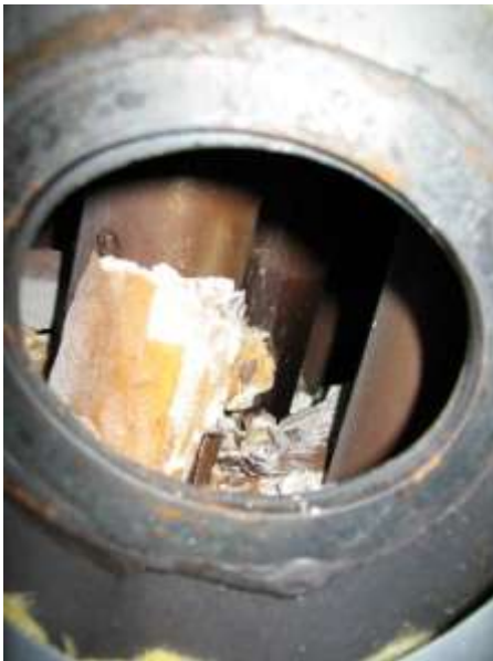
Installed 11/01/06 – room #1 out of service 02/04/08
