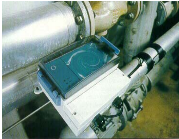
Fig 4: A typical Scalewatcher installation. Note the tightly wound coils in the centre right of the photo.
